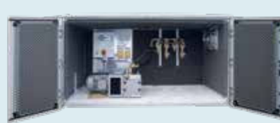
Concrete external cabinet
