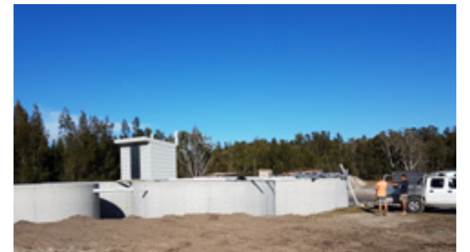
Municipal- and Industrial Wastewater Treatment Systems
