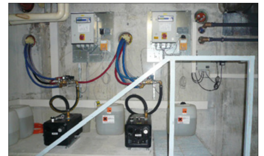
Example: Installation in an existing plant room
