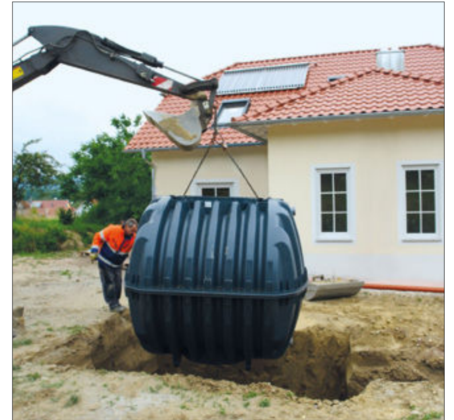
Detached house, Eichstetten (Germany)
